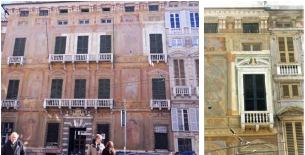
Fig. 2 Photographs at the end of restoration. The original parts of the late sixteenth century decoration were left in view around some windows of the second noble floor, found only in some parts under the next layer, painted, perfectly matching the original one, as can be seen in the details
