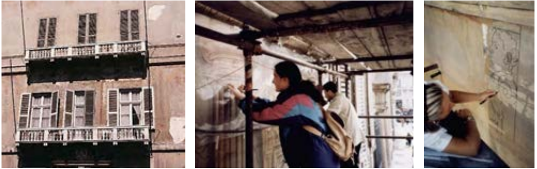
Fig.1 The facade before restoration. Survey in contact with capitals and profile hermes during restoration.
